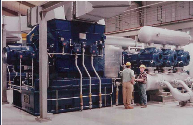
c.. VFD EMD – Gear - Compressor
