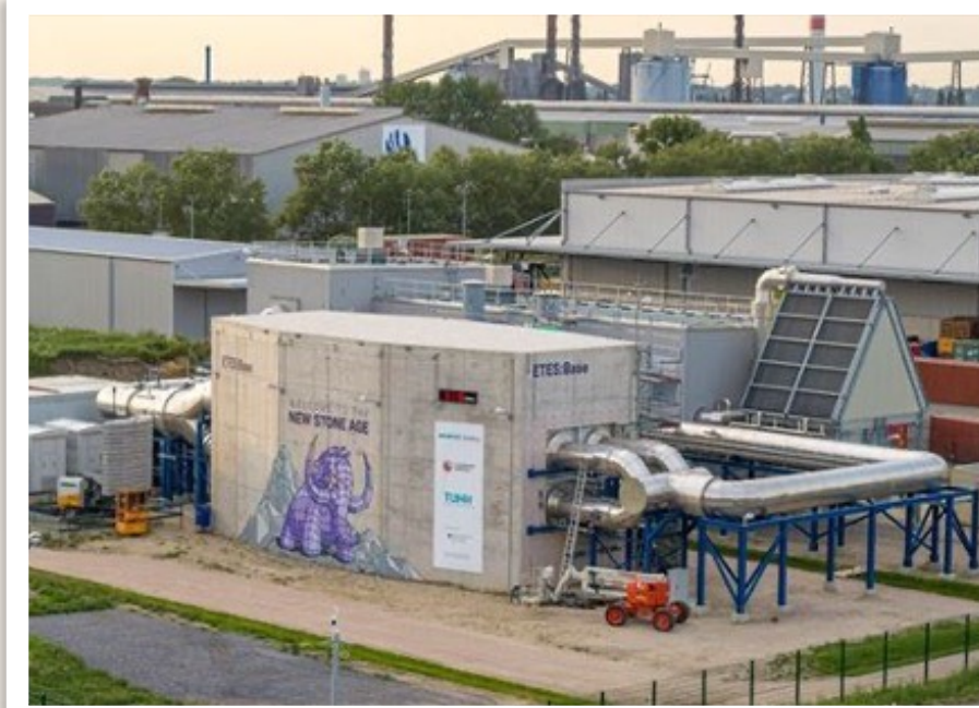
▲ ETES (Siemens Energy)
