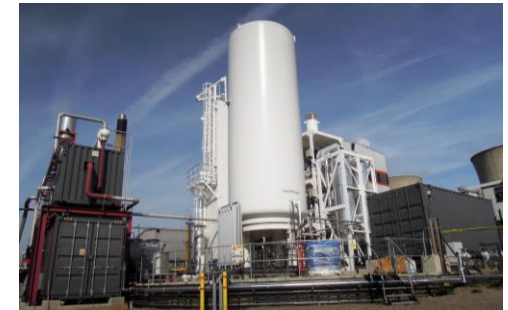
Pilot Heathrow, UK Commissioned in 2011
