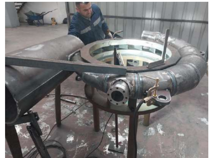
Design and build of proprietary HD turbine
